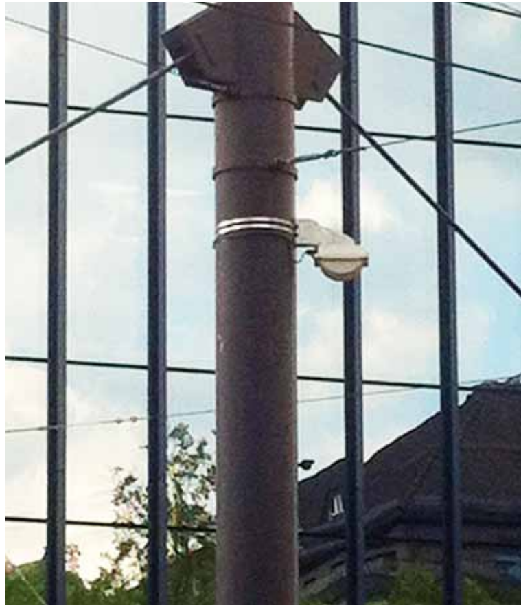
WLAN Offload Access Point in St. Gallen
